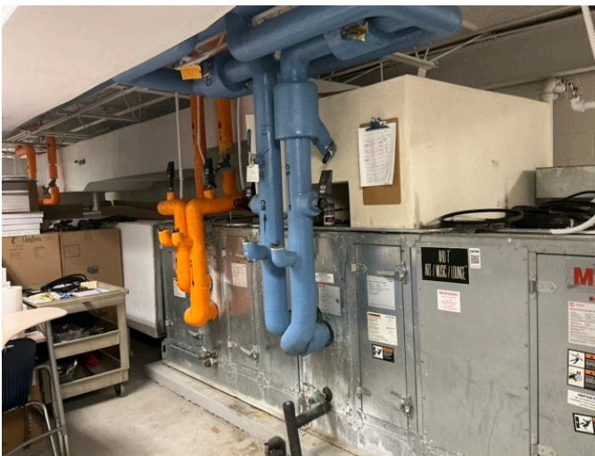
15 - SECONDARY MECHANICAL ROOM
